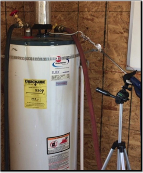
Water heater with NOx detection equipment.
