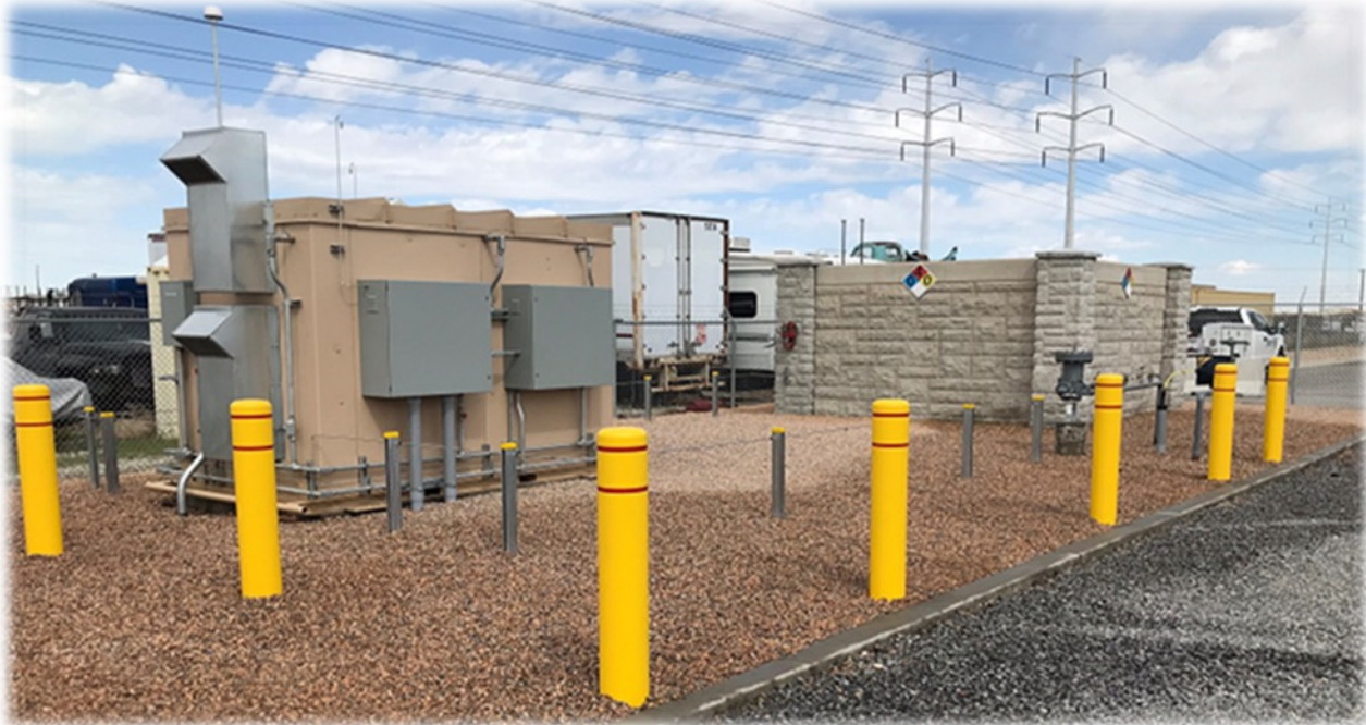
ThermH 2 – Phase 1 Facility, DEU Training Academy.
